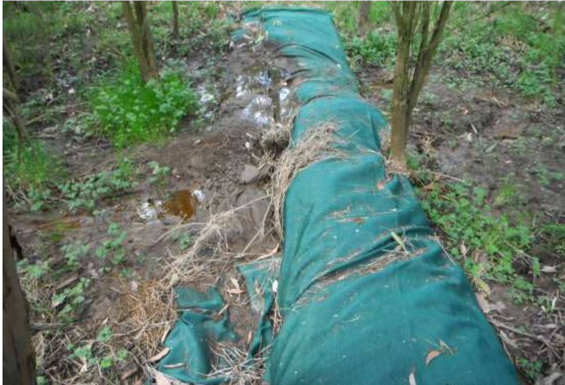
Figure 12: However, the excitement was relatively short-lived as heavier rain events overwhelmed the sediment traps and they were found to be largely ineffective under such conditions
